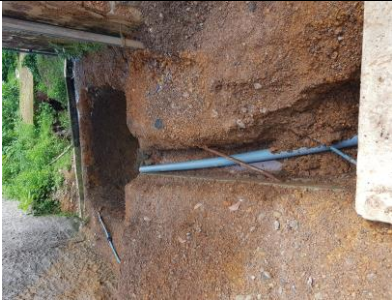
Figure 1: Uncompleted soak-away in Kenema Facility
